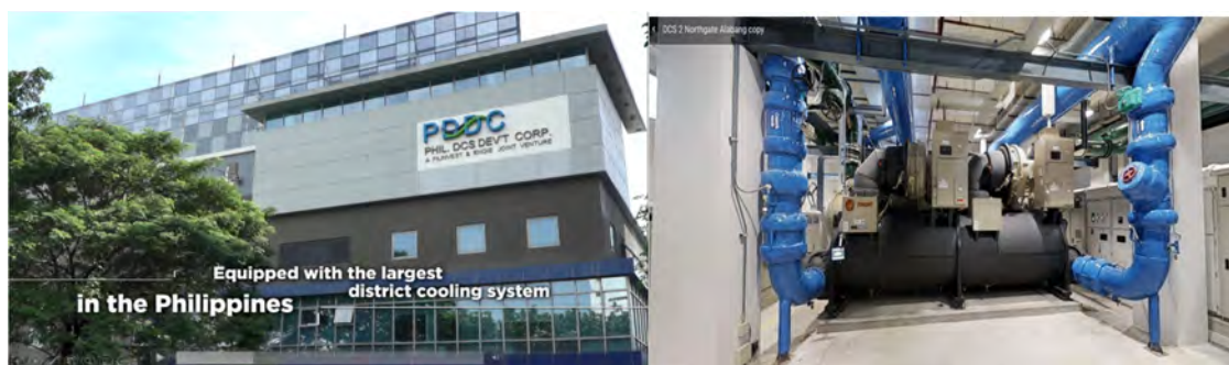
District Cooling System at Northgate Cyberzone
