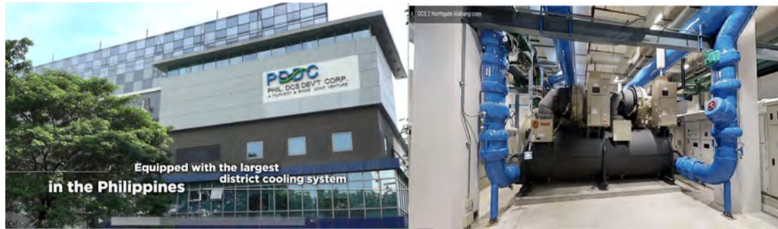
District Cooling System at Northgate Cyberzone
